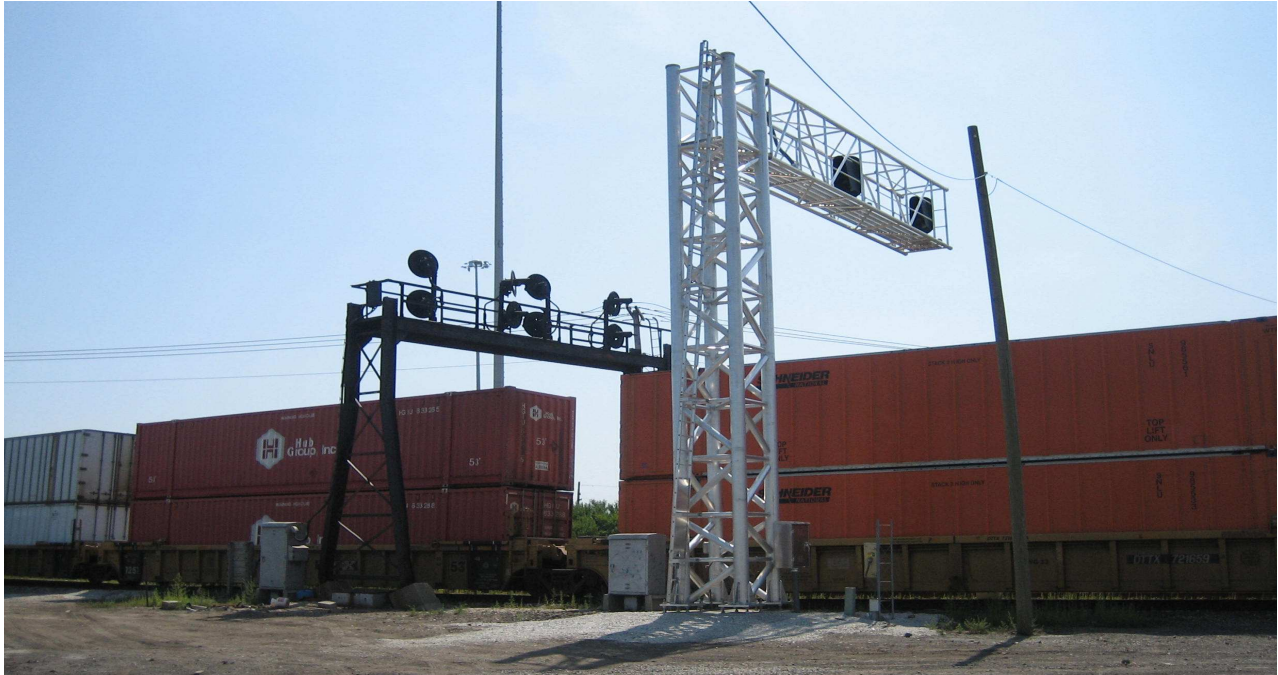
New signal bridge installed at Corwith Yard as part of CREATE improvements
