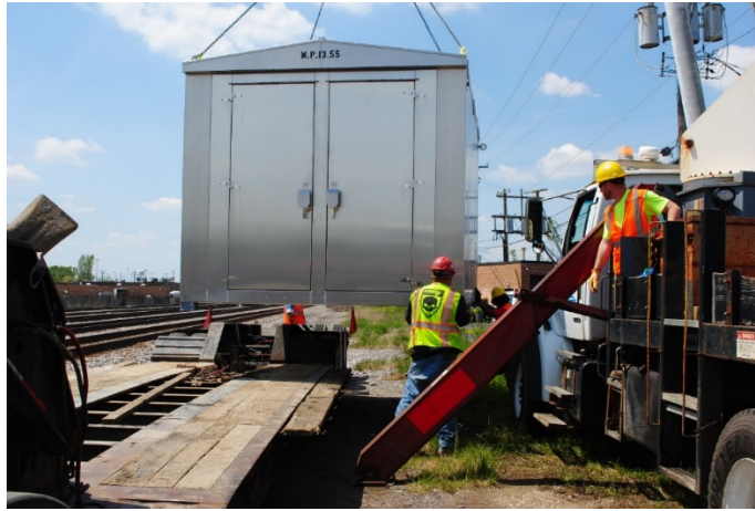
New signal boxes being installed as part of Canadian Pacific Crossover Upgrades project
